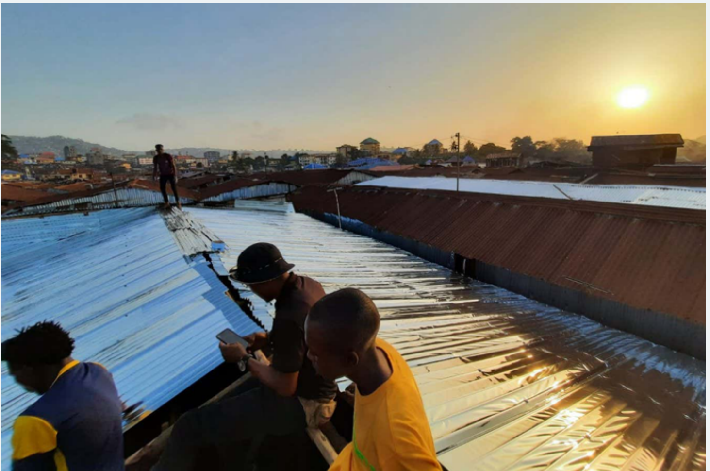
▲ Reflective film installed on the roofs of two buildings in Freetown, Sierra Leone MEER
