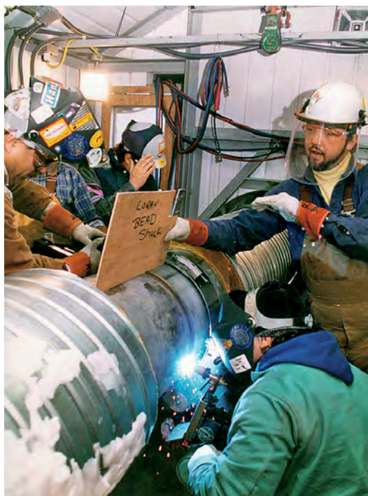
Mechanized welding of large diameter duplex stainless steel cross-country pipeline (Source: Arco Exploration and Production Technology)
