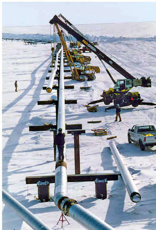
Installation of insulated 24 inch 2205 pipe on vertical support members in Prudhoe Bay (Source: Arco Exploration and Production Technology)
