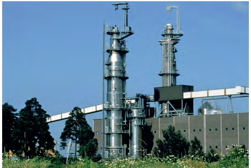
2205 continuous sulphate pulp digester and impregnation tower, Sodra Cell Mönsterås, Sweden (Source: Kvaerner Pulping)
