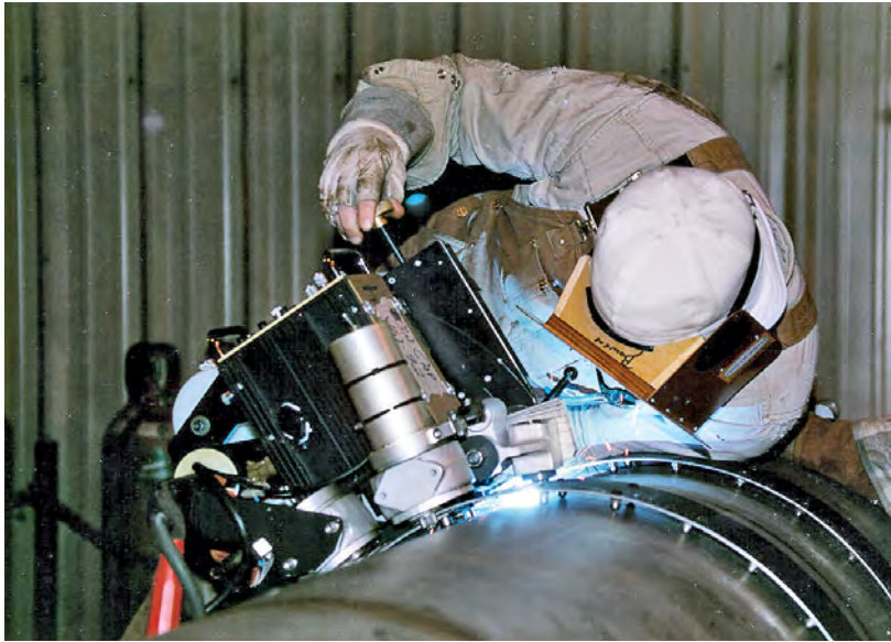
Mechanized welding of large diameter duplex stainless steel pipeline on Alaska's north slope (Source: Arco Exploration and Production Technology)
