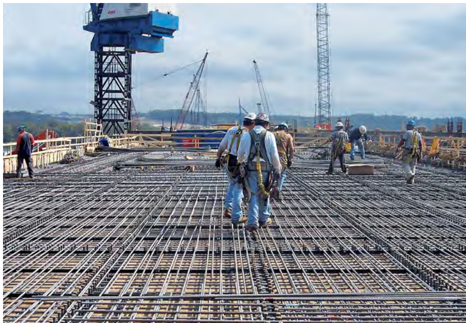
Installation of duplex stainless steel rebar on a large bridge deck (Source: Hardesty & Hanover, LLP)
