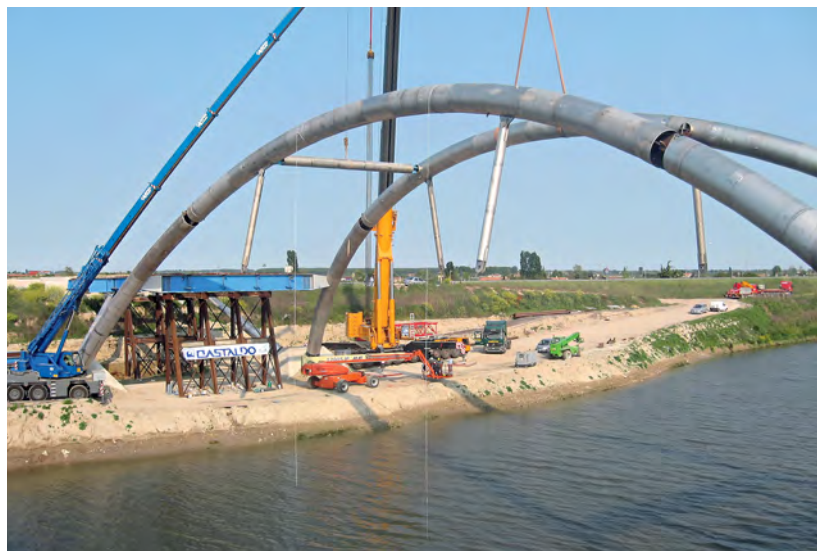
2304 duplex stainless steel bridge arches in construction near Padova, Italy (Source: ArcelorMittal)
