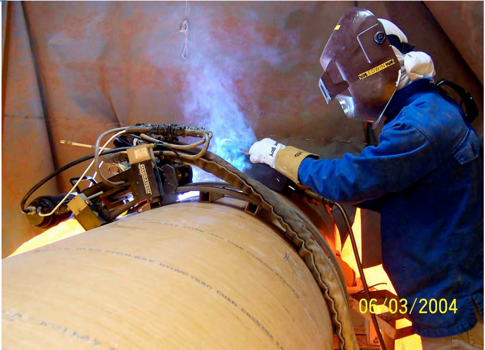
Chad - Double-Joining Pipes
