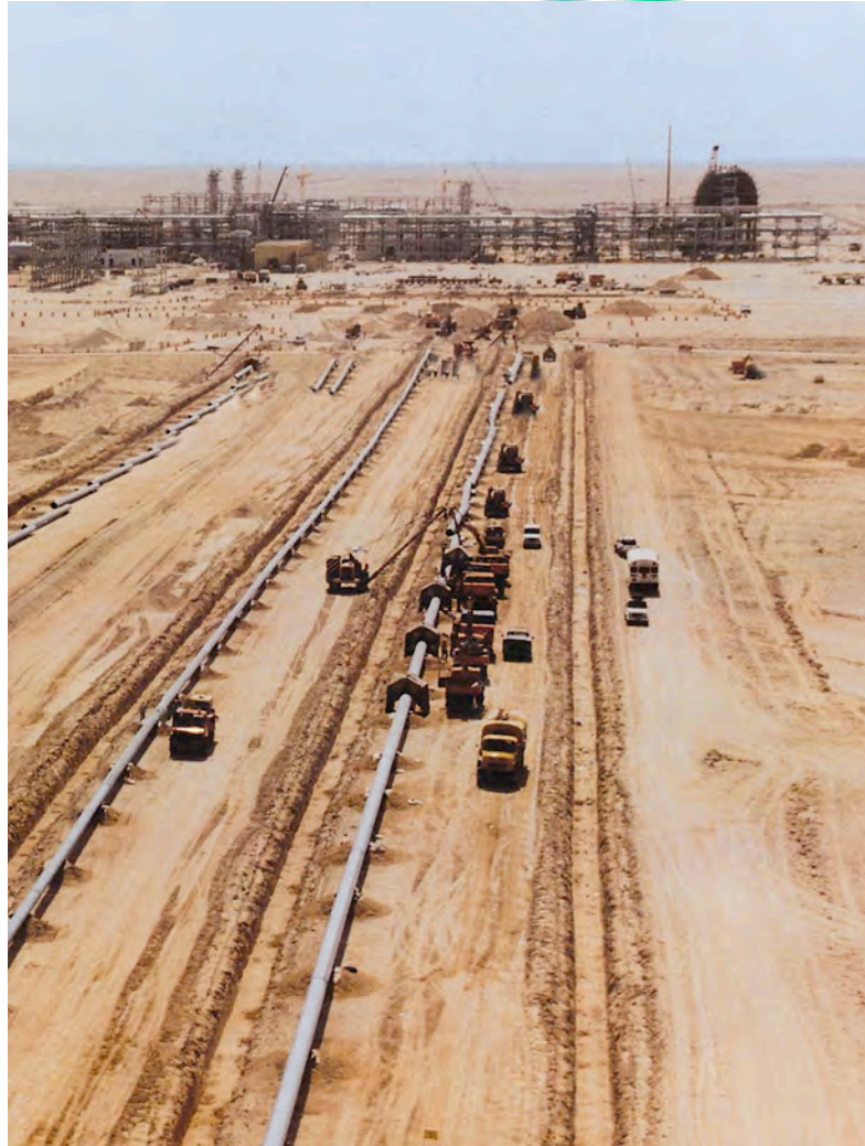
Saudi Aramco - Haradh Gas Gathering Manifold 32" x 18mm wall, X-65. 20 Pipeliner systems. Zero repair rate.
