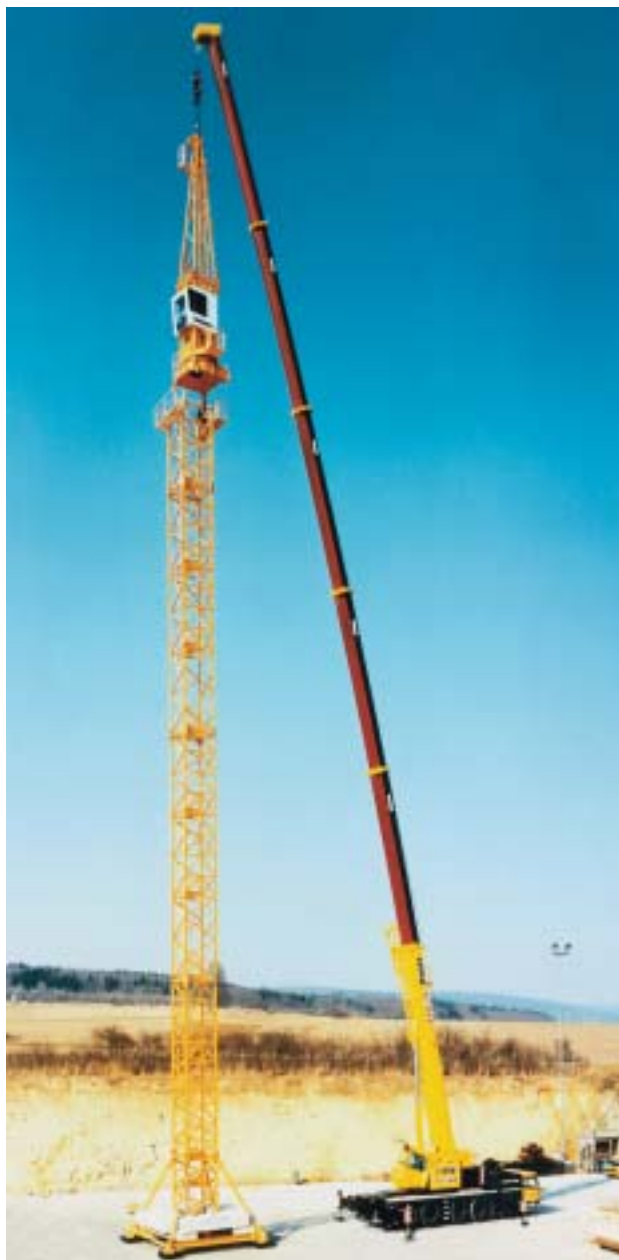
Figure 20: Mobile crane assembling a tower crane (Illustration used with the kind permission of Liebherr-Werk Ehingen GmbH, Ehingen, Germany)
