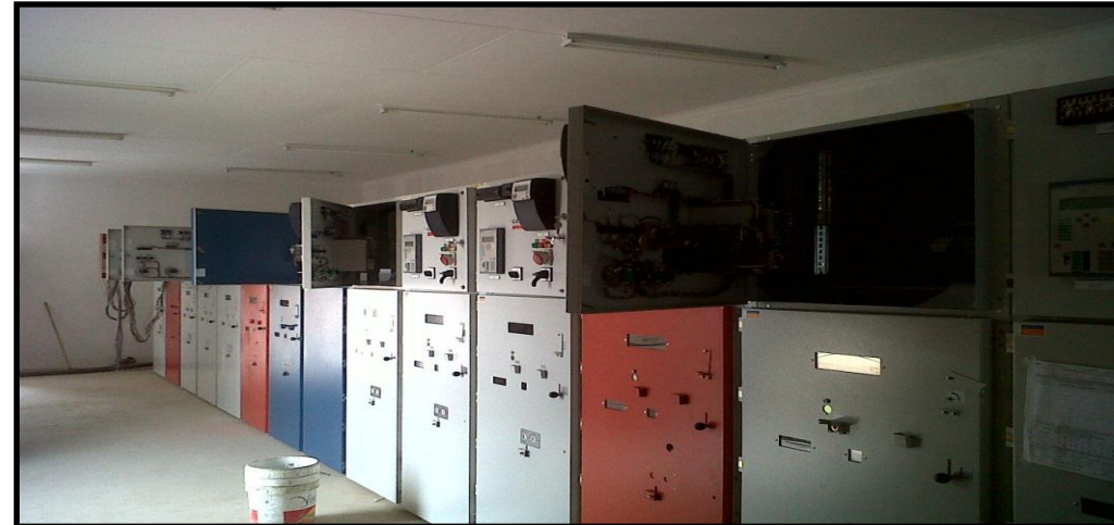
Main consumer substation: switch room
