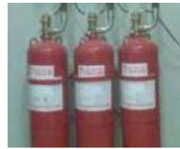
NITIE 1230 Fire Suppression System
