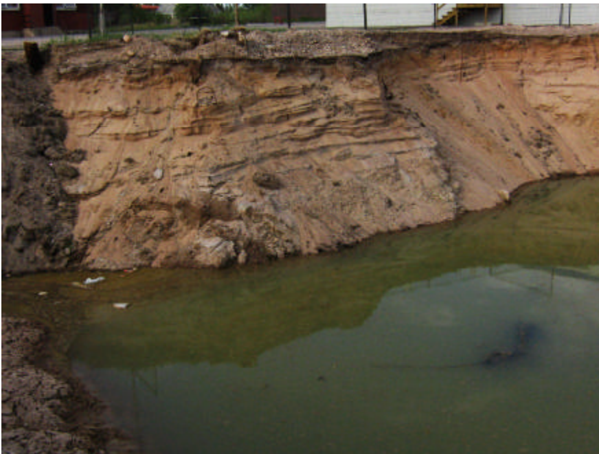
Figure 12. Part of the excavation to remove sands contaminated by diesel fuel in Fort Chipewyan. 2 June 2007.
