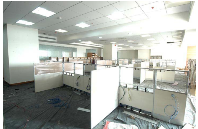
Exhibit 10: Fit-outs were ongoing in January Anant Raj Manesar IT park site in January 2010
