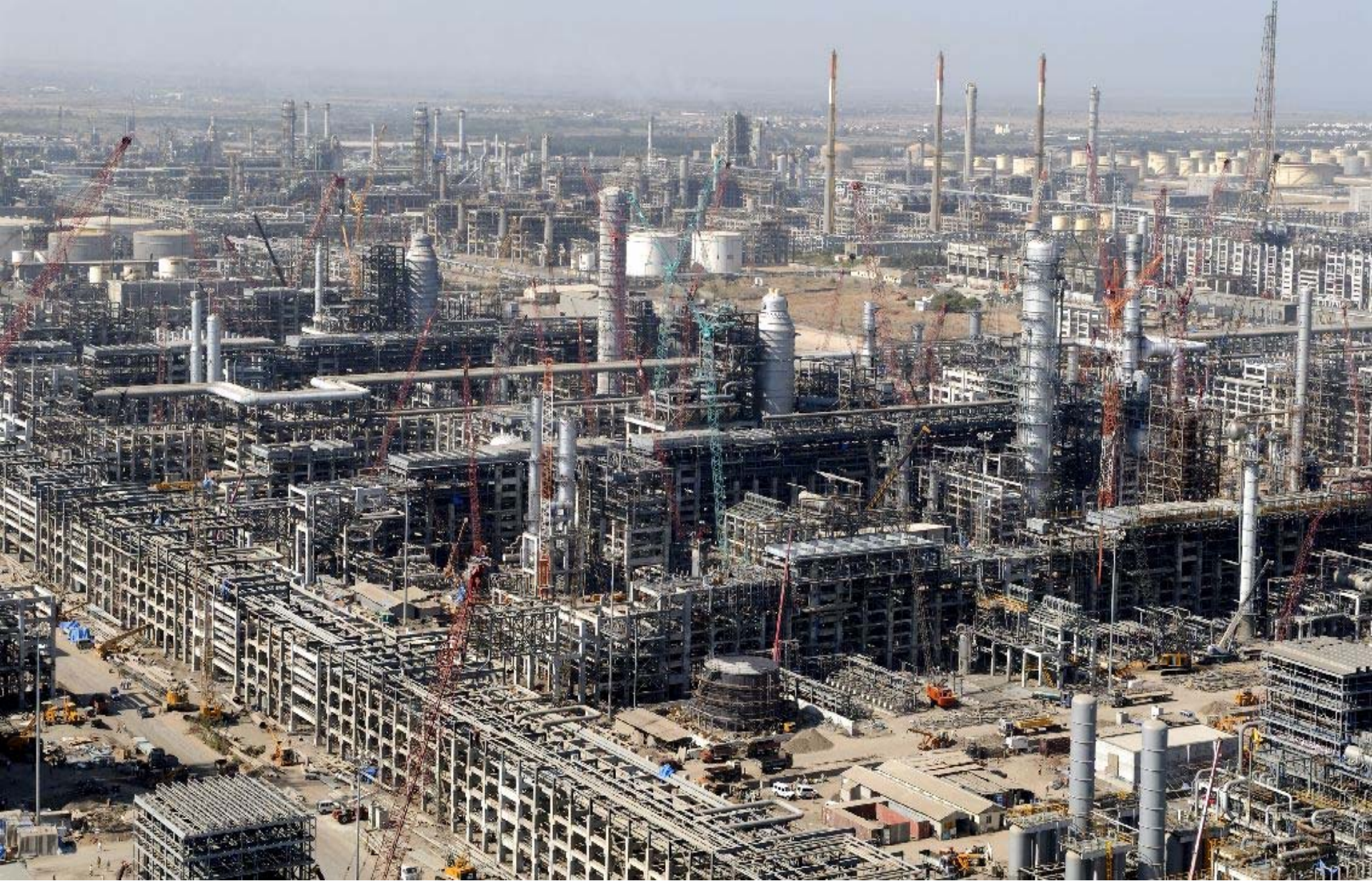
Overview of the Crude Complex
