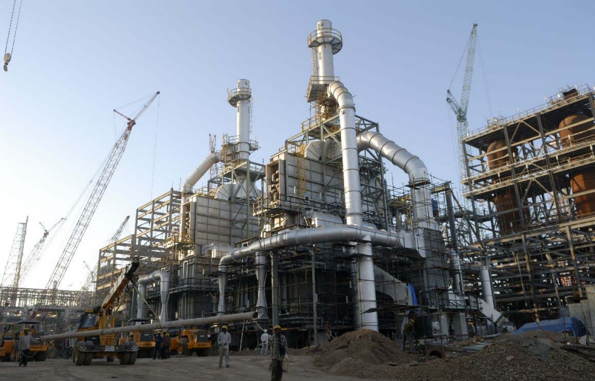
Overview of the Diesel Hydro De-Sulphurization (DHDS) unit
