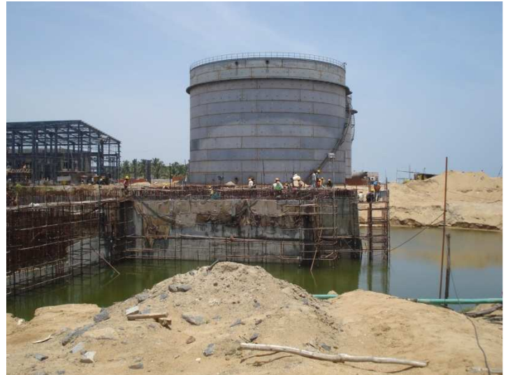
EXHIBIT 21: Ultrafiltration filtrate storage tank
