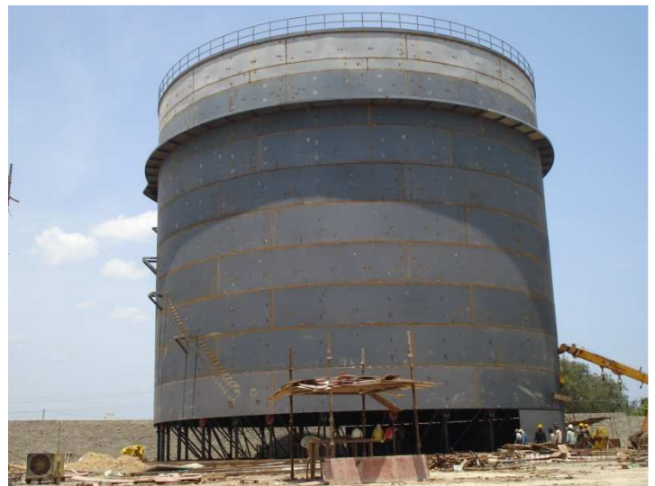
EXHIBIT 23: Reverse osmosis filtrate storage tank
