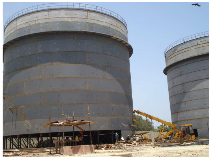
EXHIBIT 25: Filtrate storage tanks
