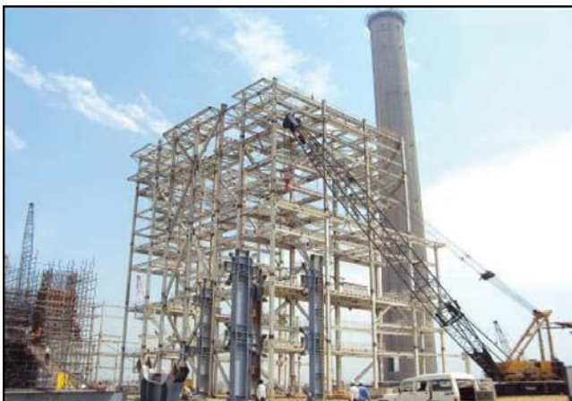
Exhibit 53: Boiler erection in progress at Tiroda 1 st unit (660 MW) Site photograph of Tiroda 1 st unit
