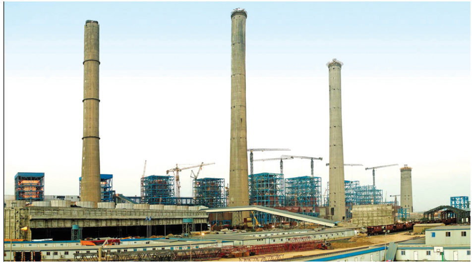
Exhibit 51: Chimney erection completed for all the 4 phases of Mundra project Site photograph of Mundra phase I-IV
