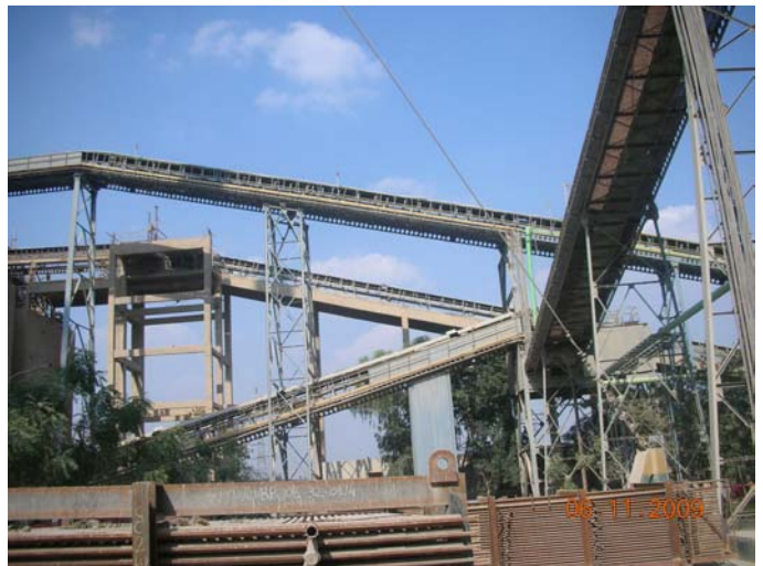
Fig 16 - Conveyor belt to move clinker
