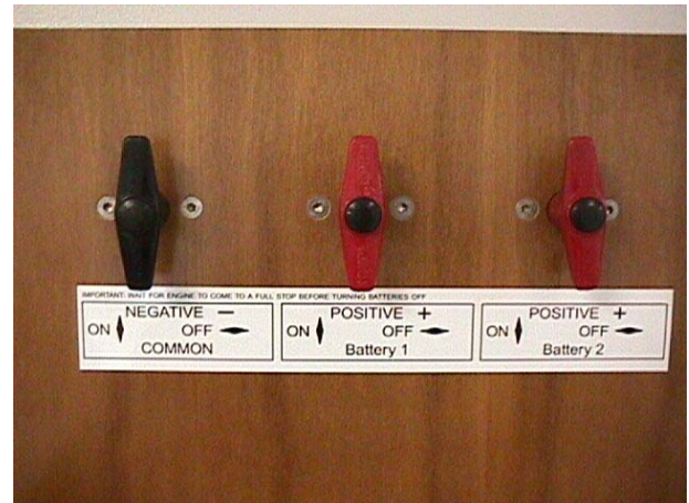
Everything is ON, 12VDC power available to start engine and/or run equipment
