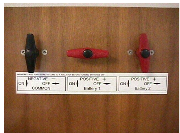
Engine is off , Run equipment from house only ( like at anchorage)
