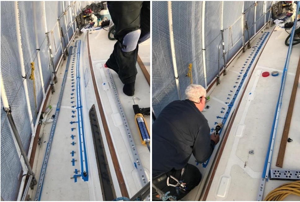
Checked every captured fastener hole to make sure it would all lock down tight. We used SikaFlex 295 UV bedding compound. Cleanup excess spouge was a real PITA.
