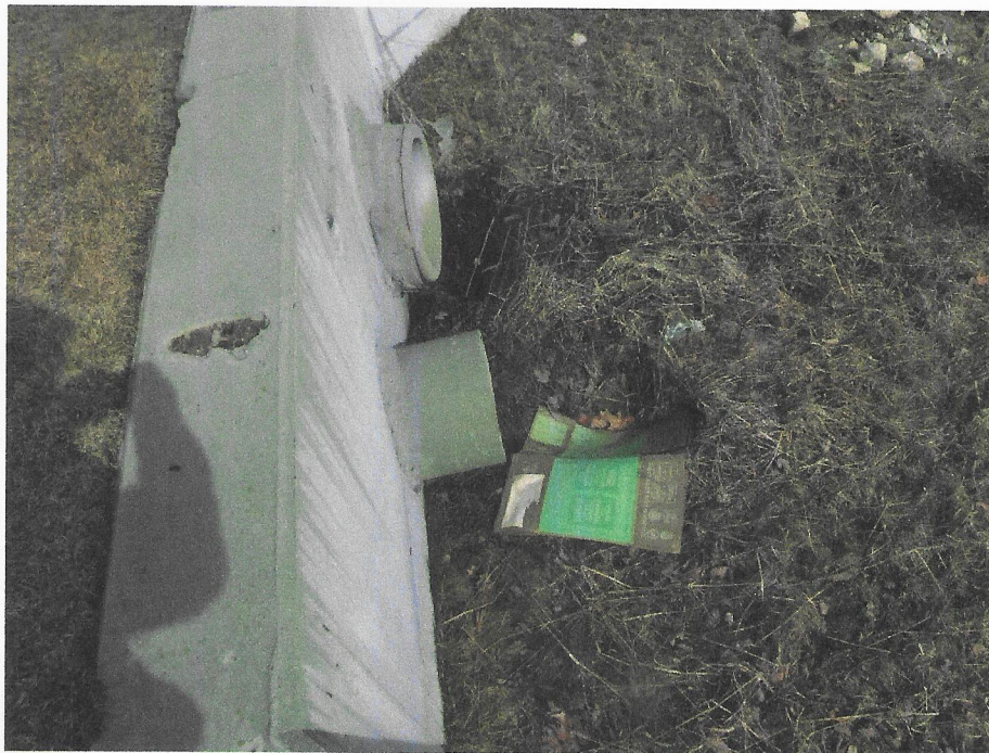
Erosion at outfall between lots 11 & 12
