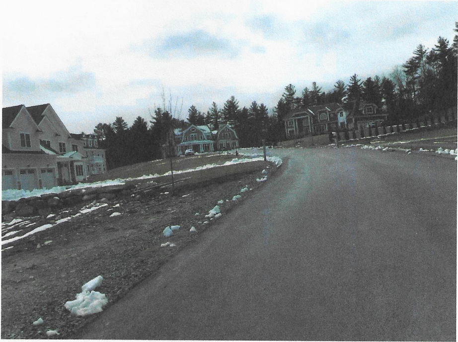
Crushed stone swale along edge of road at Lot 11 and 12 to be re-established
