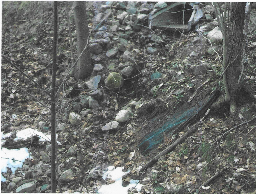
Bank erosion at outfall from DMH-1 Additional Rip Rap needed
