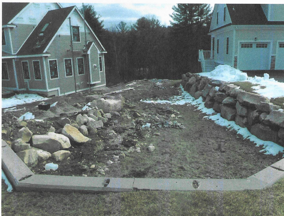
Swale and check dams between lots 11 and 12 need to be constructed
